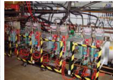
power amplifiers (TWTs)
